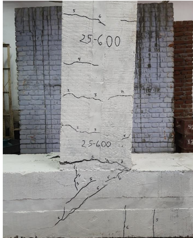
Figure 3.48: Cracking characteristics of joint reinforced with B600C-R
